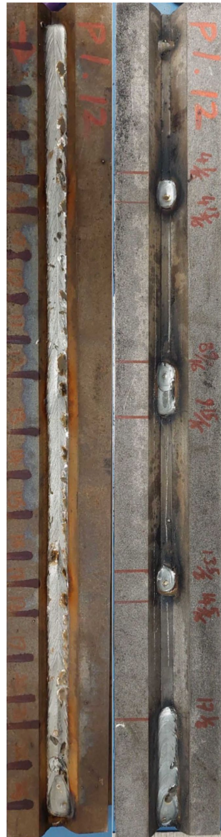
Fig. 11 A consistent, uniform weld bead (left) achieved across varying root openings, gaps, and diverse tacks within the joint (right), without prior information or pre-scanning provided to the robot
